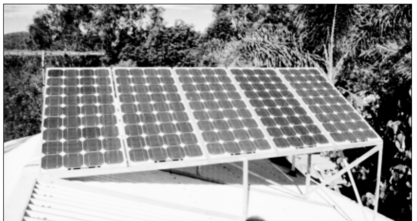
BELOW: Our home power supply five x 80 watt solar panels. On a house you have the advantage of being able to set the panels up at the correct angle to the sun for maximum output. Made all the better with no mast or rigging to shade them
