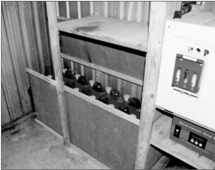
LEFT: 6 x 2 volt x 1100 Amp hour batteries make up our home power storage. A 1200 watt Selectronics Inverter supplies our 240 volt needs including running tools for building my new boat
