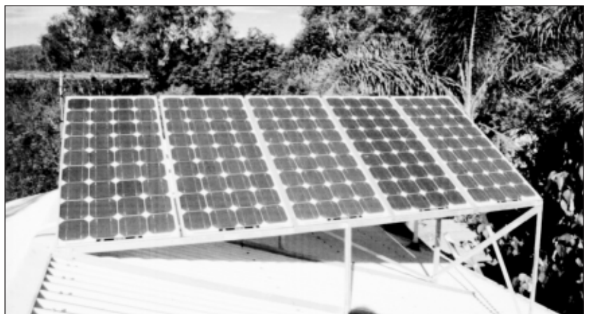
BELOW: Our home power supply five x 80 watt solar panels. On a house you have the advantage of being able to set the panels up at the correct angle to the sun for maximum output. Made all the better with no mast or rigging to shade them
